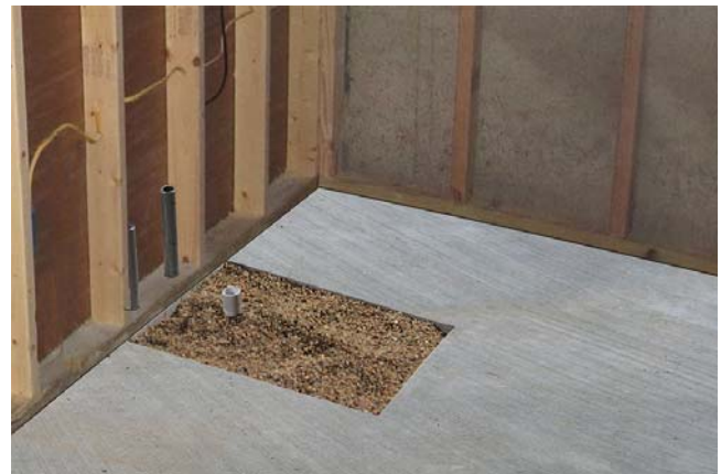
Particle Barrier used to block termites from entry at bath trap
