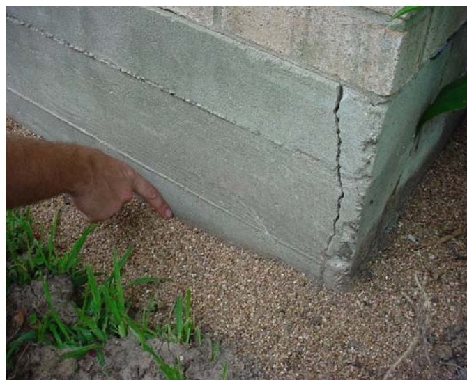
Pointing to a place where Reticuletermes flavipes were blocked from leaving a structure to replenish moisture
